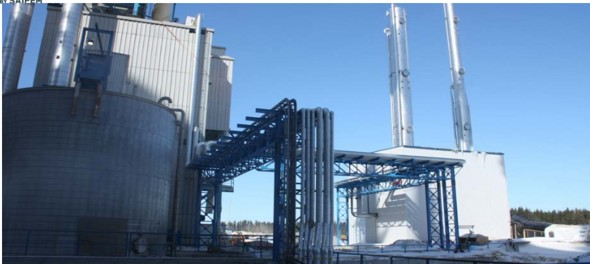
CO2 Capture Plant of 30 tons per day operating on a commercial scale at Saint-Felicien, Quebec, Canada
