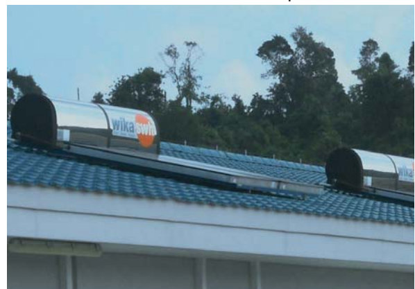
Solar panels in Karimun
