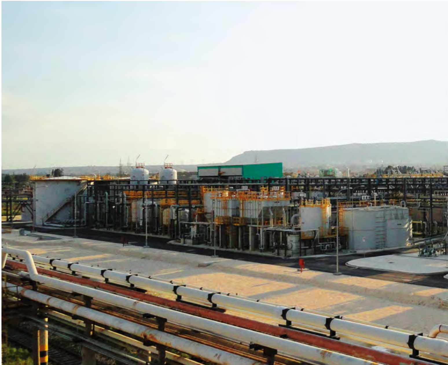
TAF project in Priolo - Italy: Overview of the groundwater treatment plant with a capacity of 600 m 3 /h
