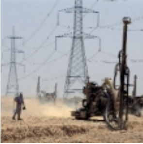
Saudi Arabia, excavation of a trench for the laying of a pipeline.
